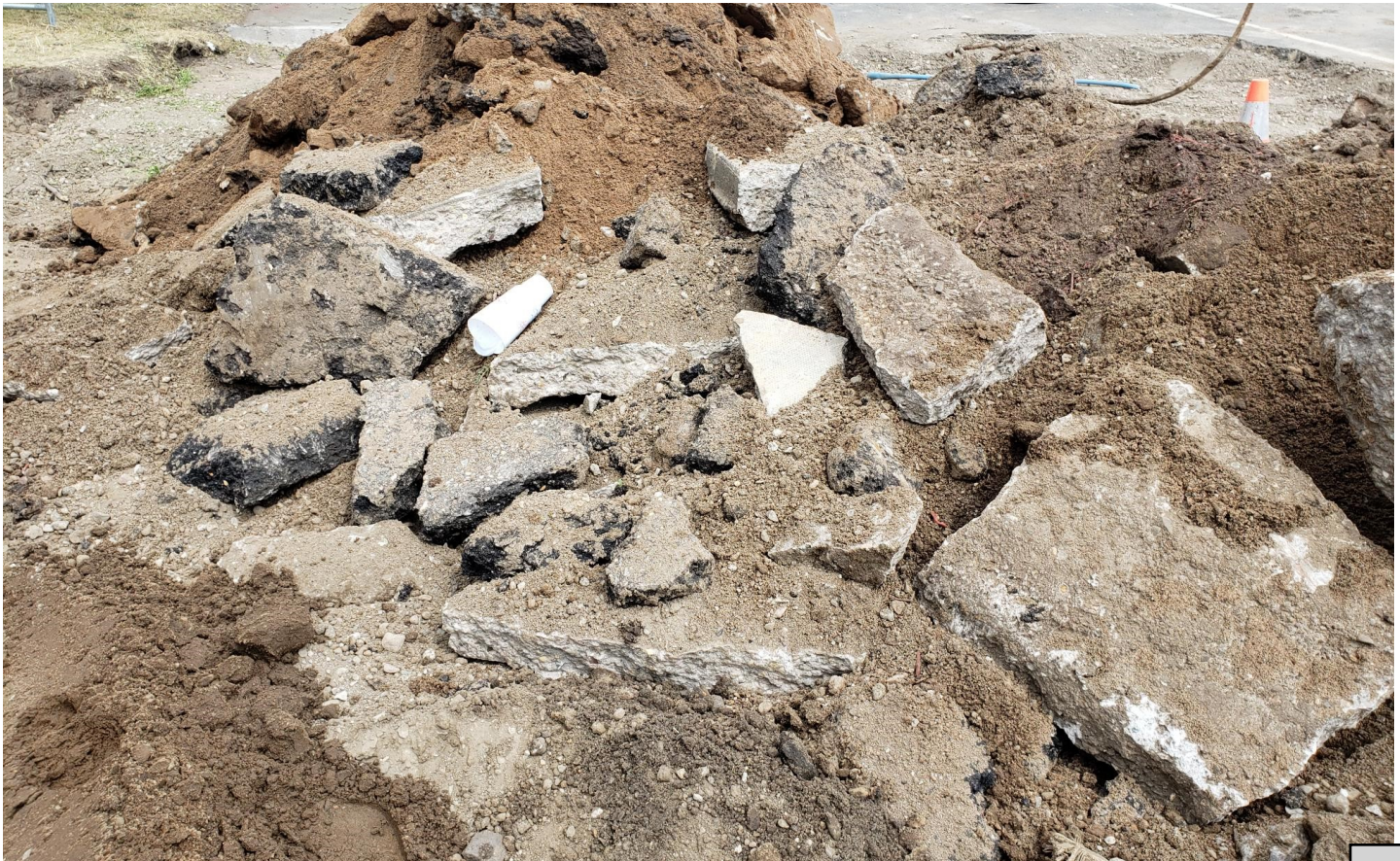
Above: Concrete debris buried within limits of new lift station
