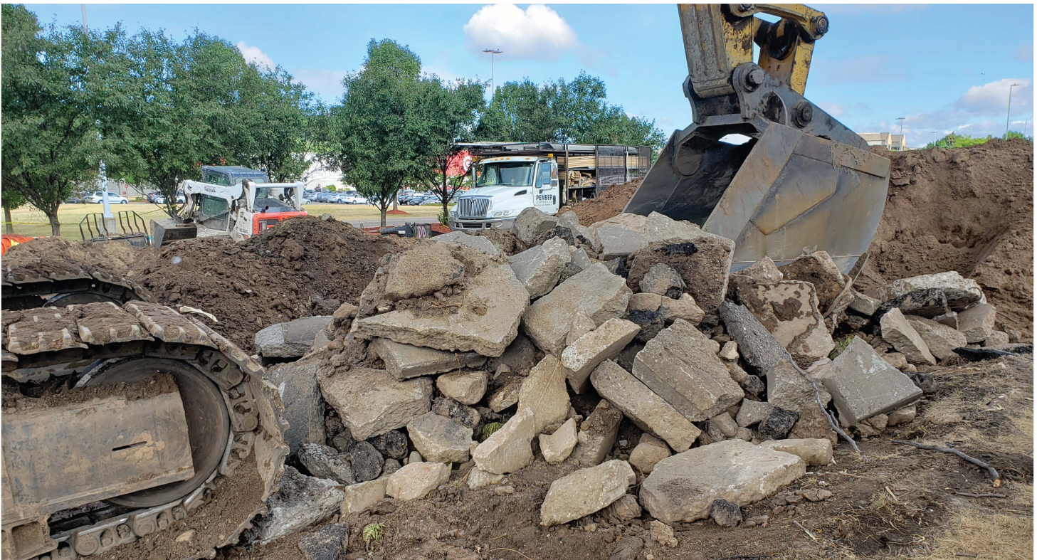
Above: Accumulated debris encountered within utility corridor
