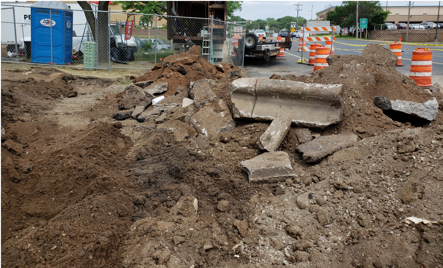
Above: Concrete debris buried within building and utility corridor
