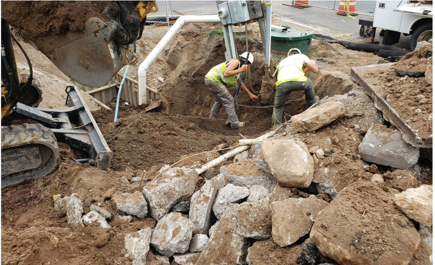
Above: Buried concrete debris near existing lift station along 53rd Avenue
